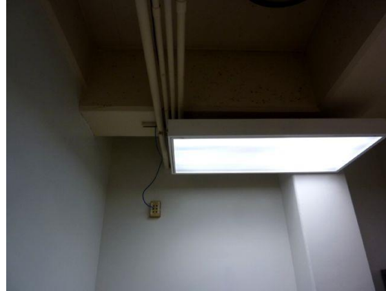
Level 2 DC Power Panel Circuits in Storage Overhead
