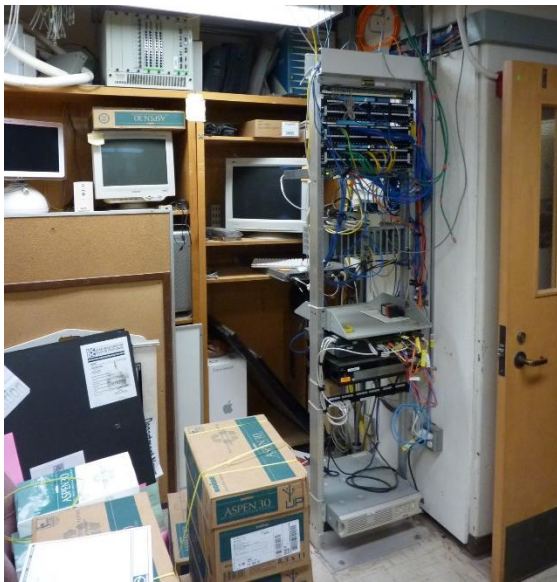
Level 1 Storage IT Rack
