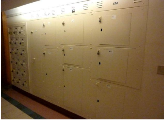
Level 1 Electrical Panelboard in Corridor
