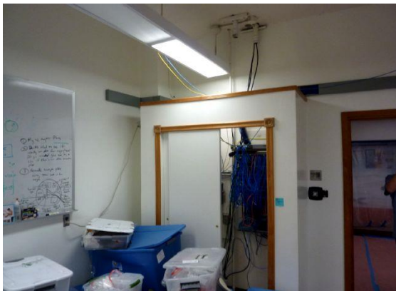
Level 2 IT Closet
