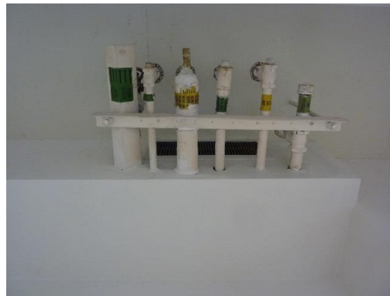
Level 1 Office Plumbing Piping Stubbed Services
