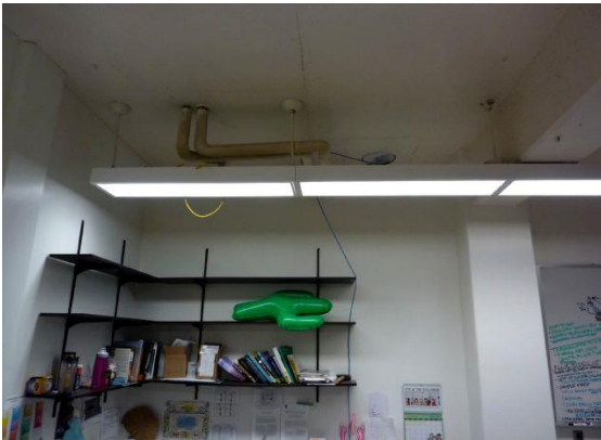
Level 2 Lab Overhead Piping
