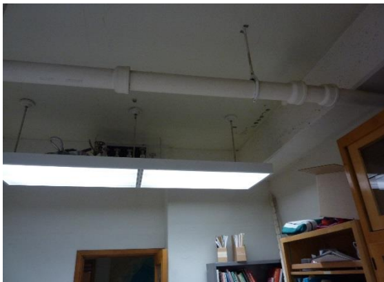
Level 1 Office Industrial Waste Piping
