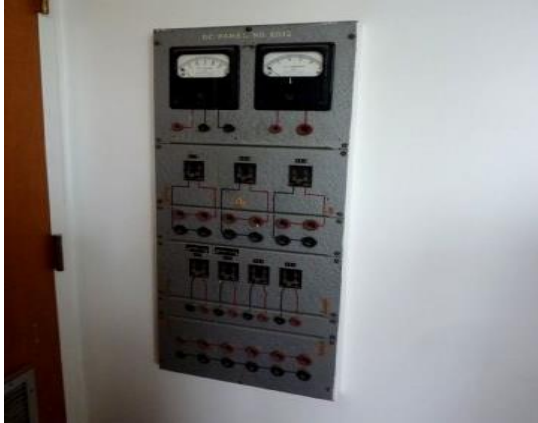
Level 2 DC Power Panel
