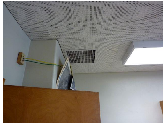
Level 2 Office Telecomm Cabling
