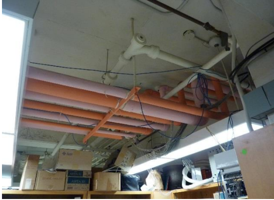
Level 1 Receiving/Storage Plumbing Piping Mains
