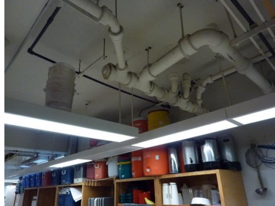
Level 1 Receiving/Storage Industrial Waste/Vent Piping
