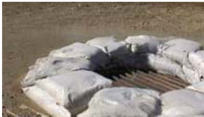
Figure 3 Gravel Bag Barrier for Street Stormdrain Inlets
